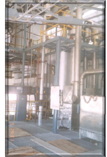
Gas Cleaning Unit
