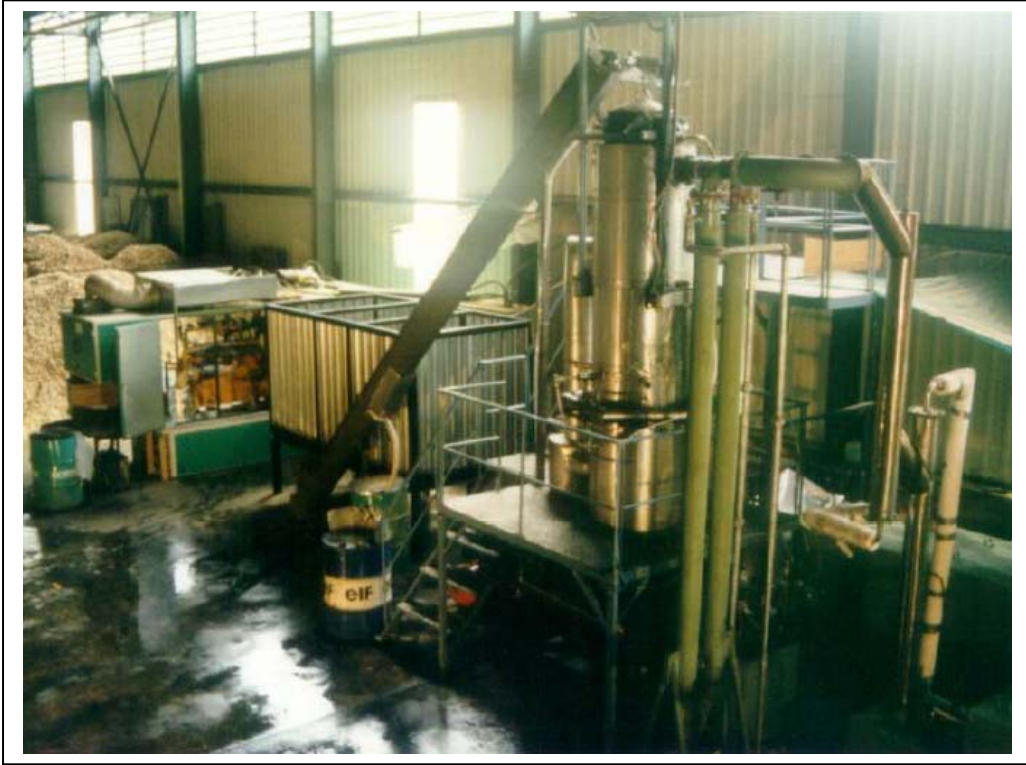
The 100 kg/hr Gasifier at Switzerland
