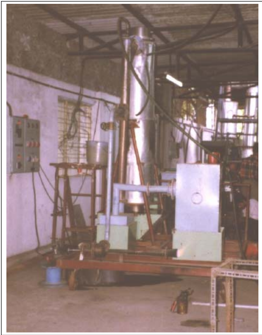
A 3.7 kWe Gasifier, test setup at the laboratory
