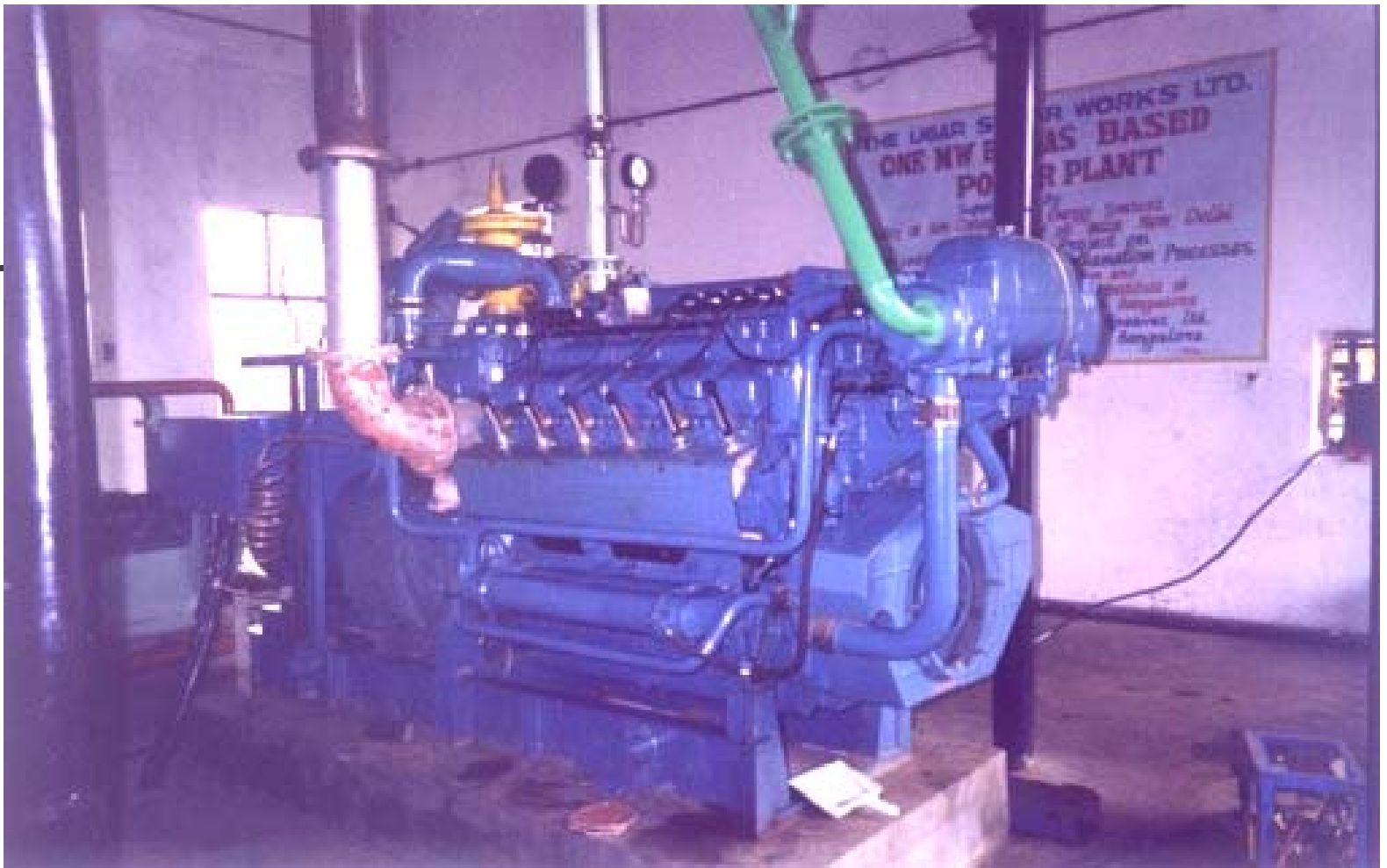
Picture of One of the Four Greaves Engines of 300 kVA Capacity Installed at USWL
