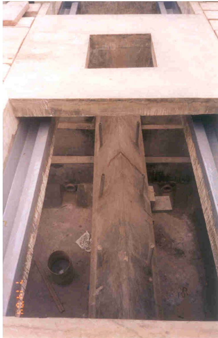
FEED INLET POINT & DEFLECTOR BEAM
