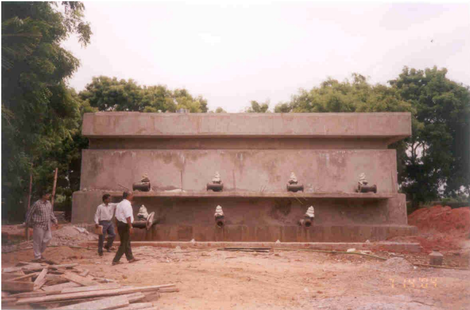
SLUDGE WITHDRAWAL PIPES
