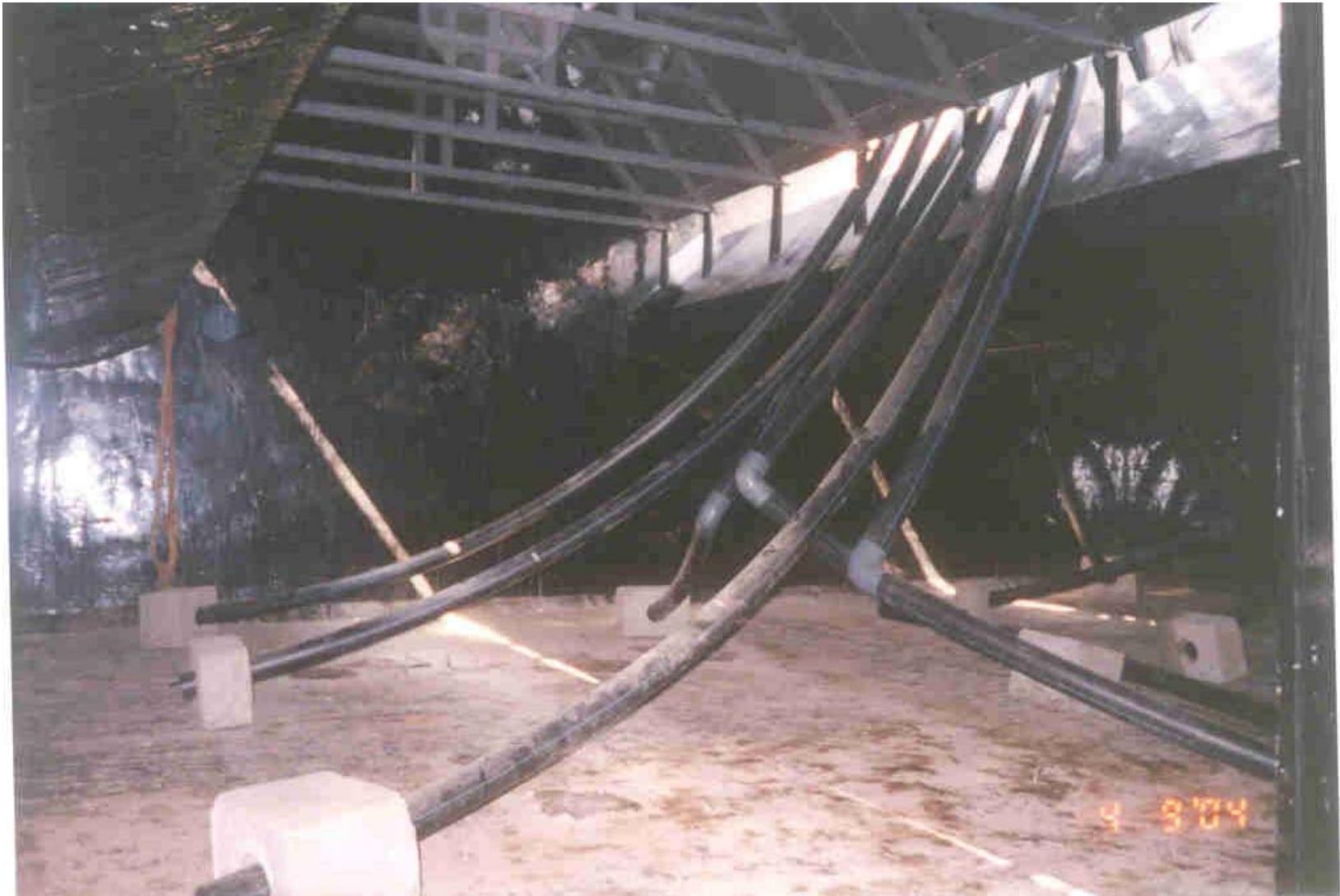
FEED INLET PIPES IN UASB
