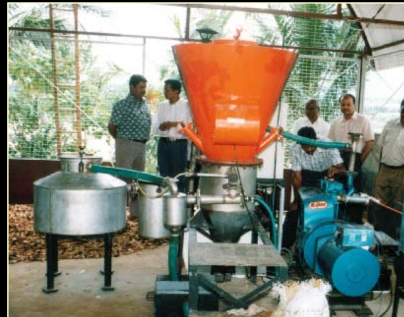
Gasifier Model: 1 X GAS-9 Odanduthurai, Coimbatore
