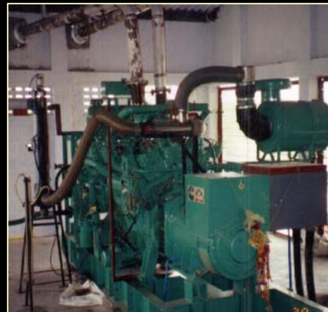
System Package : GAS-200
