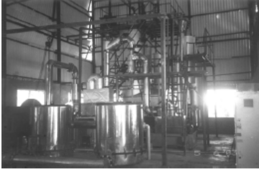
Figure I: The gasification system at M/S Hindustan Pencils, Jammu
