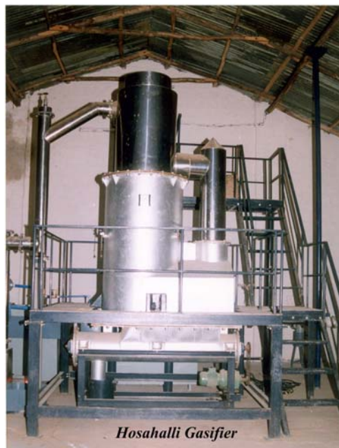
Plate 1: 20 kWe Biomass Gasification System at Hosahalli, Karnataka
