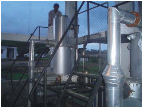
2 x 10 kWe Gasifier System at Kasai
